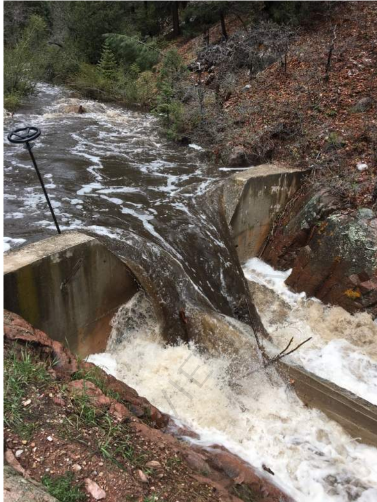
Figure 5 – May 2017 Flow at Beulah Water Works District Raw Water Diversion
